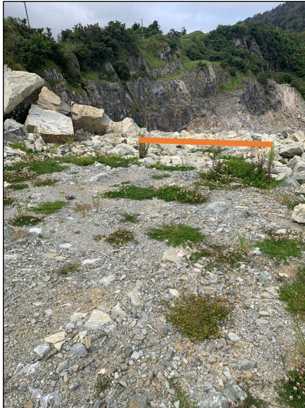
Photo Four - Missing Open Edge Protection (orange line)
